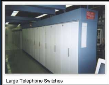
Large Telephone Switches
