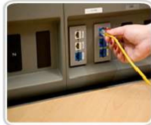
Cables must be connected correctly.
